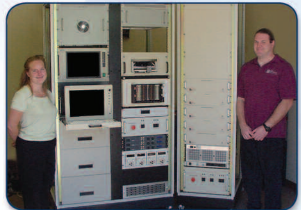
NTS developed the Test Adapter Test Set (TATS) for L3 Communications in order to provide field maintenance testing of avionics components of a helicopter based Anti-Submarine Warfare System.
